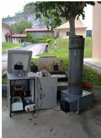
Fig. 2: PV-battery-inverter unit connected to the Belonio rice husk gasifier. PV module tilt angle shown for illustrative purposes only.
