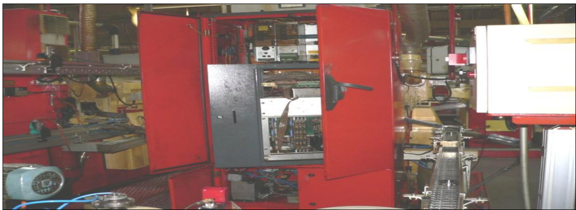
Figure 1: Electrical cabinet at workshop
