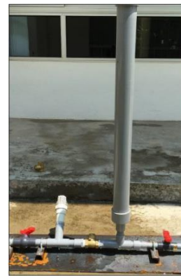
Figure 4. Adjustable waste valve installed at hydram
